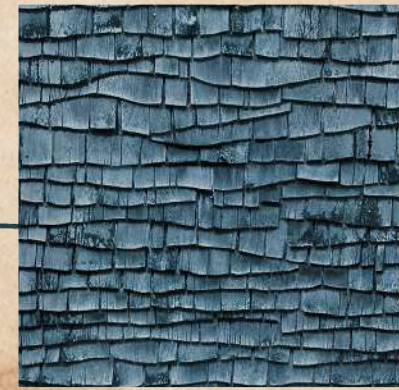
Broken Wooden Shingles
